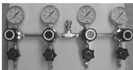
four-regulator panel with center inlet
